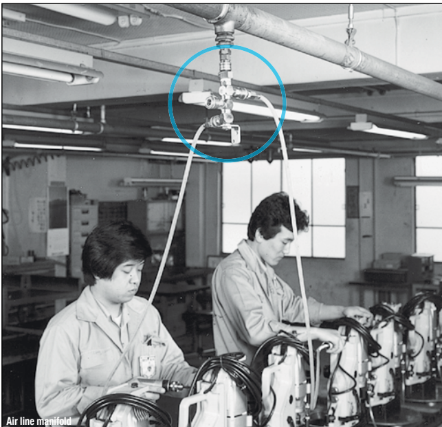
Air line manifold
